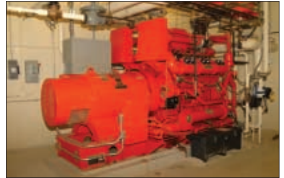
Above: This Waukesha VGF L36GLD powers a Trane chiller to help keep classrooms comfortable at the West Campus of Pima County Community College in Tucson.
